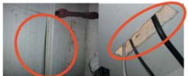
Examples of damage to the metal cladding caused by impact damage
